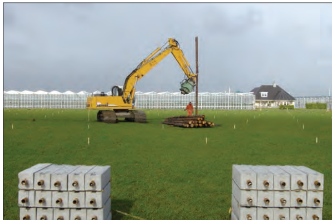
Figure 3: Timber piles being driven into soft ground using the arm of an excavator (to be followed by vibro-driving). Square section concrete extensions are in the foreground
